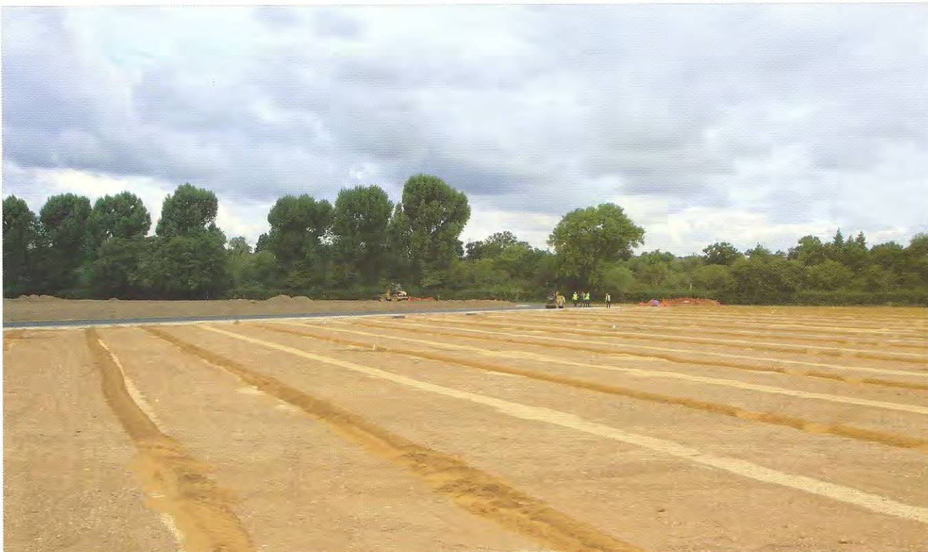
Three metre drainage bands across one of the new rugby pitches (above); below: Agripower's Gary Plummer uses a dual-grade laser for levelling the cricket square
